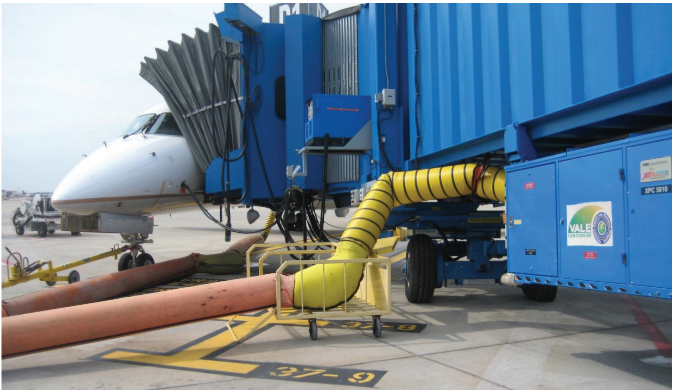
Pre-conditioned Air and Ground Power Units.
