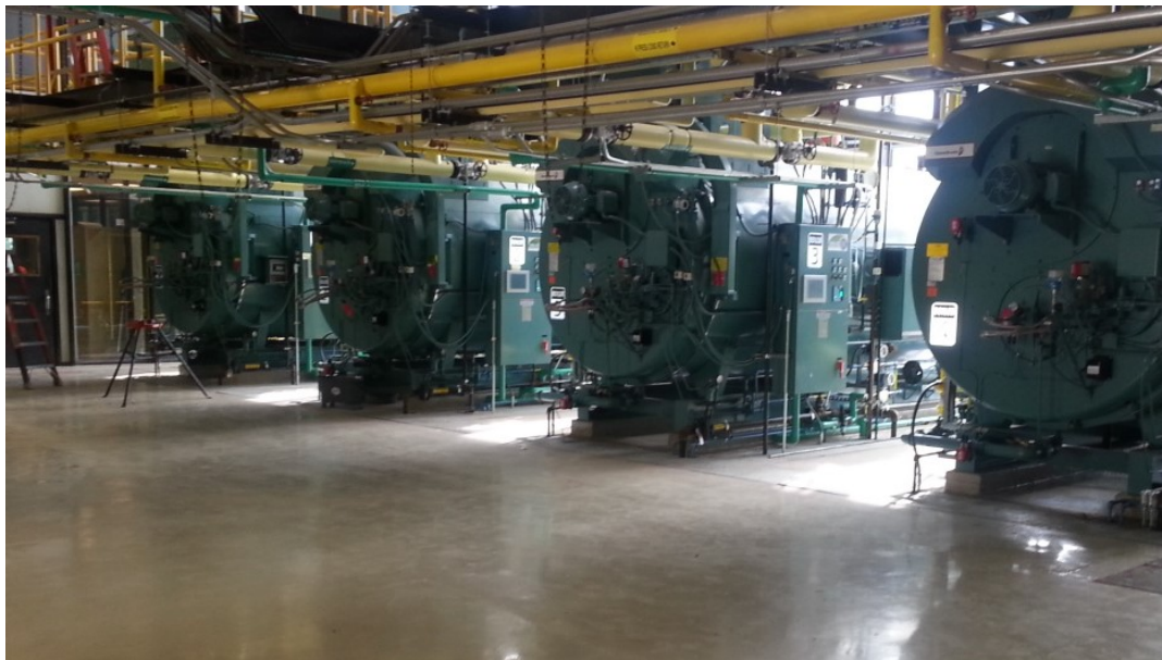
Figure 6. High-Efficiency Natural Gas Boilers in Central Power System for the North Terminal
